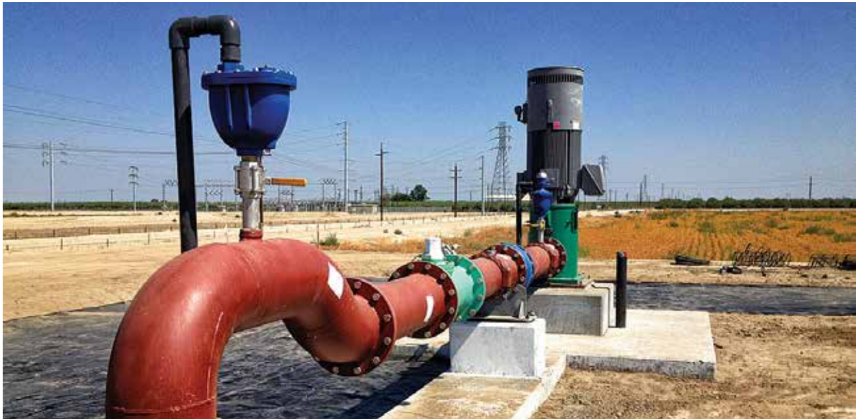
Strand Ranch Water Banking Pump
