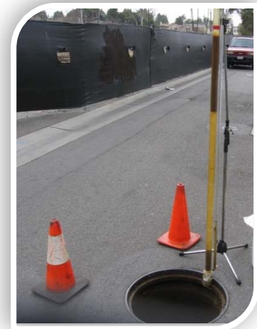
A Probe is Used to Measure the FOG Accumulation in a Grease Interceptor
