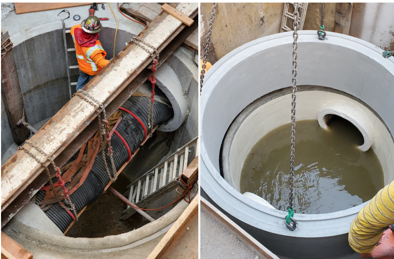
Grit Trap constructed in live flow on 42-inch RCP sewer upstream of Siphon S10 as part of the Phase 1 Sewer Siphons Project.
