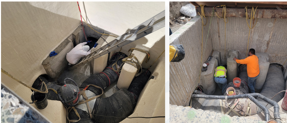
Flow-through plugs installed at S2 siphon structures to provide flow bypass during vault and siphon barrel rehabilitation work as part of the Phase I Sewer Siphon Project.
