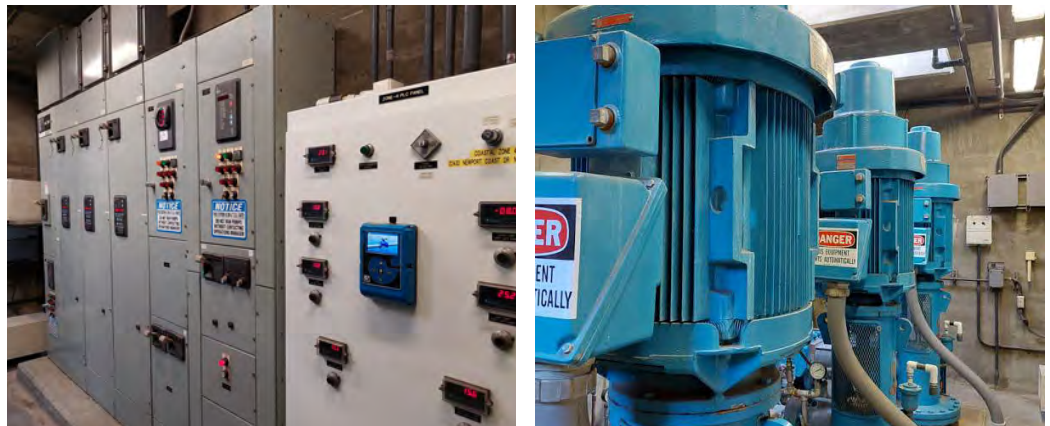
Figure 1: Existing pumps, electrical, and instrumentation at the CZ 2-4 lift station
