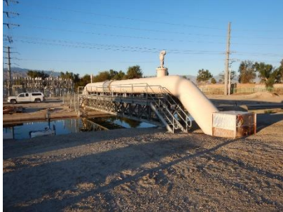
Steel Pipeline belonging to CVWD
