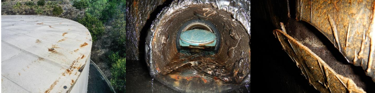
Corrosion on tank roof
