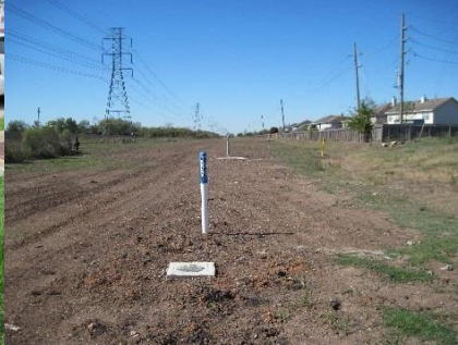
At-grade Test Station
