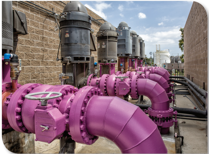
IRWD Recycled Water Pumps. Michaelson Plant, Irvine.
