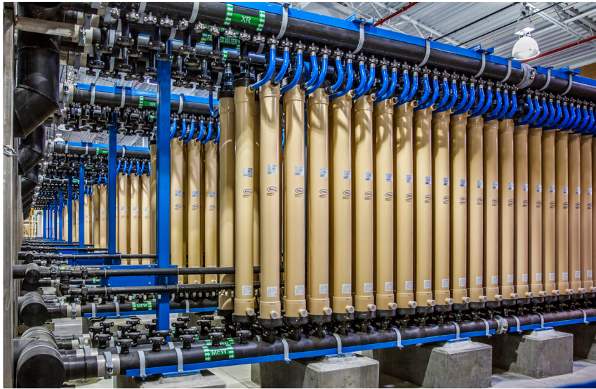
Microfiltration tubes inside the Baker Water Treatment Plant, a 28.1-million-gallon-per-day drinking water treatment facility in Lake Forest. The plant was a joint regional project by five south Orange County water districts and went online in early 2017. The Baker Water Treatment Plant is managed and owned by IRWD.
