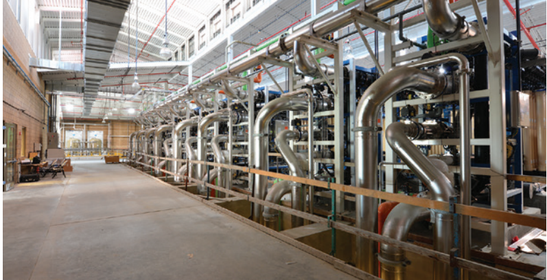
Baker Water Treatment Plant
