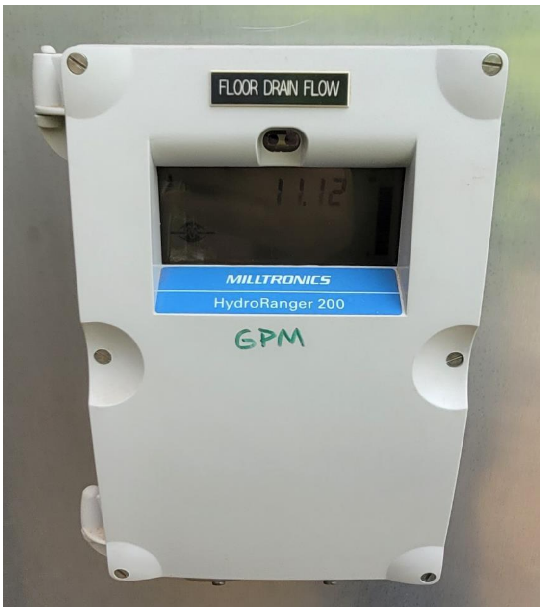
Photo 1: View of the floor drain seepage showing 11.12 GPM.
