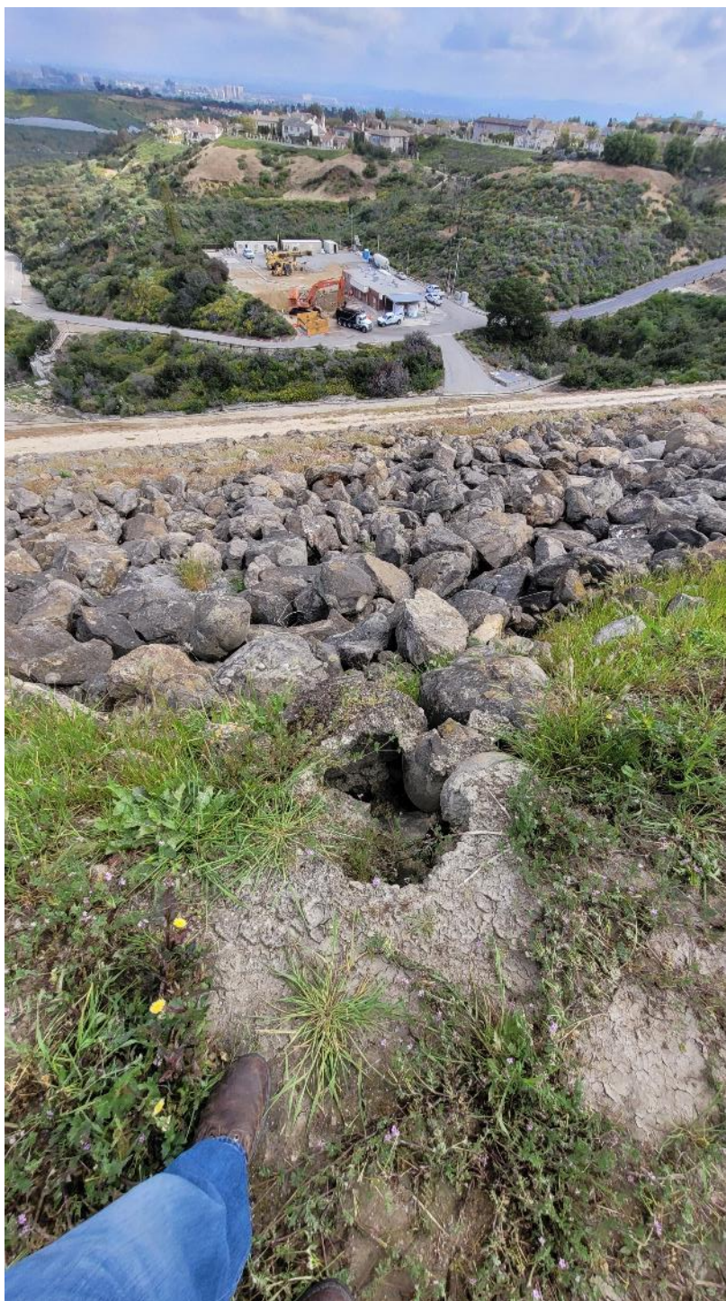
Photo 2: View of the erosion rill on one of the downstream benches.
