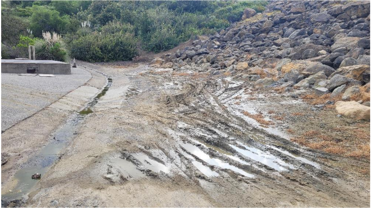
Photo 3: View of the seepage and rain collected at the toe of the dam.
