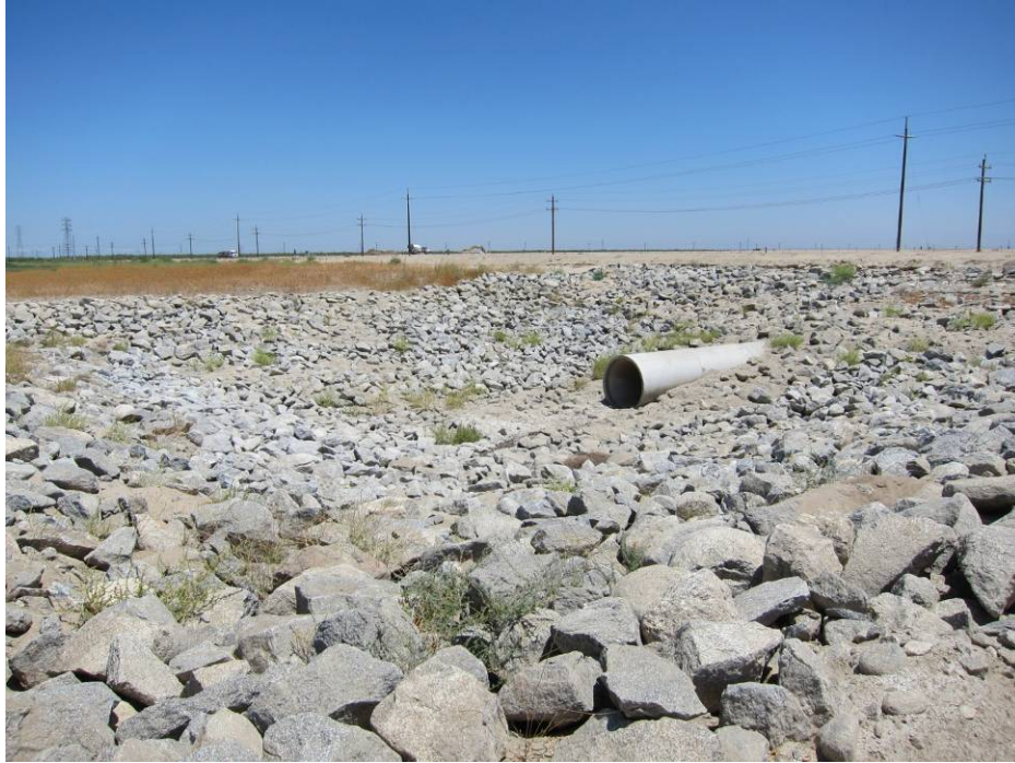
Photo 7 – Photo depicts the culverts associated with the water recharge basins on the Stockdale West property
