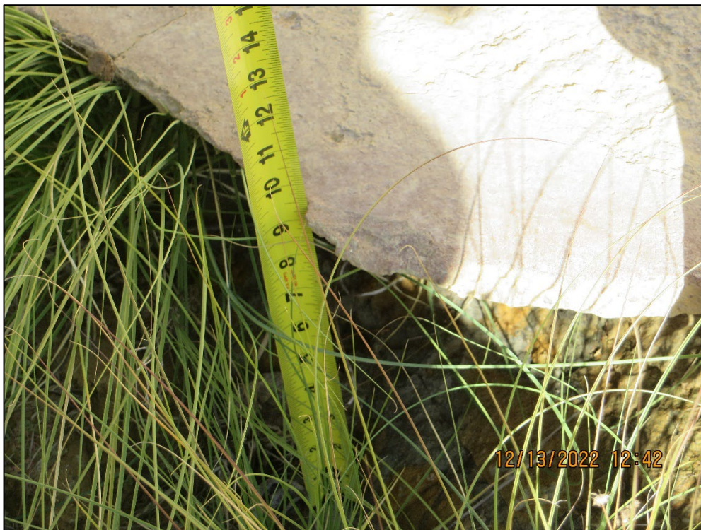
Photo 14) Close up view of undermining of recent concrete repair. Undermining is approximately 9-inches in height.
