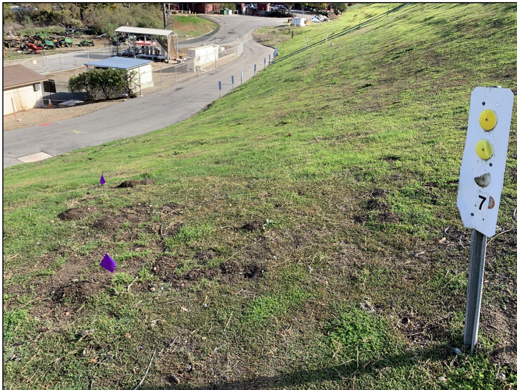
Photo 6) Downstream face looking towards the right abutment. Note signs of rodent activity and flag markings.
