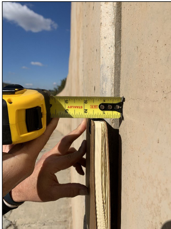
Photo 10) Approximately 1-inch vertical wall joint offset.
