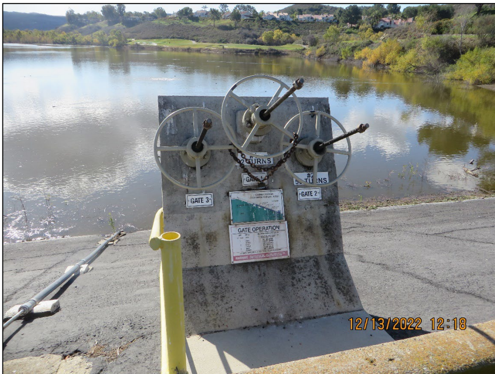
Photo 16) Outlet valve controls and stems.
