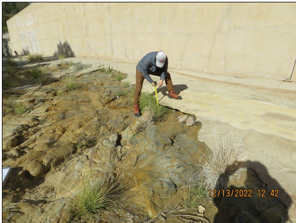
Photo 12) Looking downstream at undermining of previous localized concrete repair areas.
