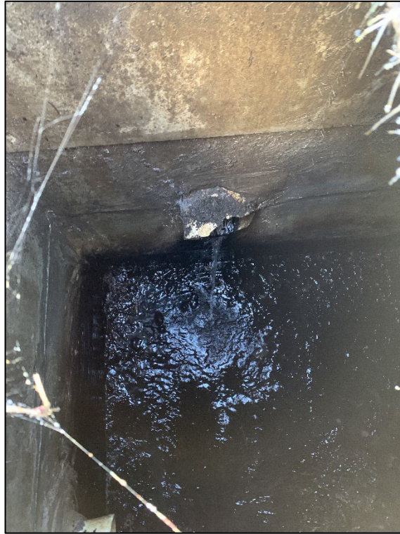
Photo 19) Seepage at left subdrain.
