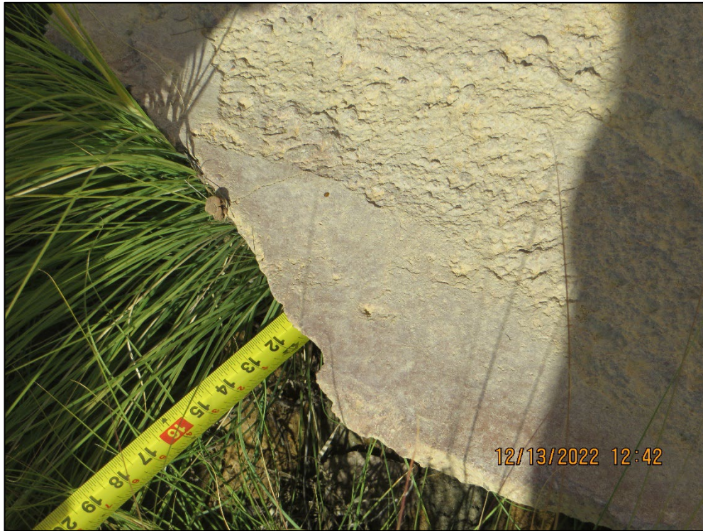
Photo 13) Close up view of undermining of recent concrete repair. Undermining is approximately 12-inches wide.
