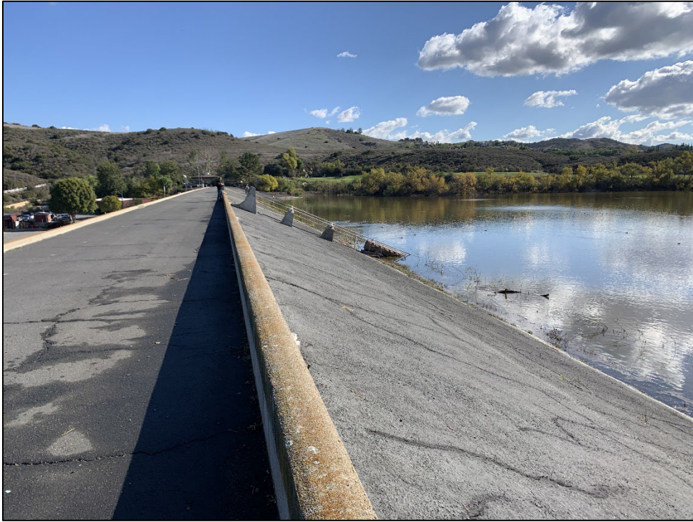
Photo 3) AC-lined upstream face looking towards right abutment. Note cracks and brush in reservoir.
