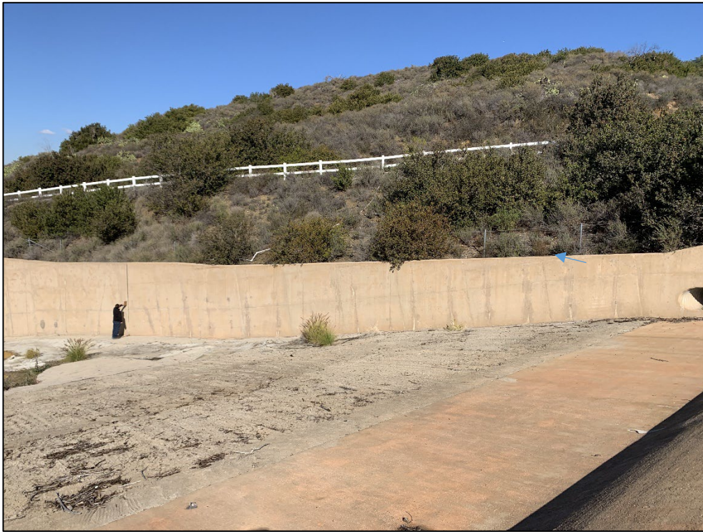
Photo 9) Spillway channel looking east. Rich Sanchez is inspecting vertical wall joint offset.
