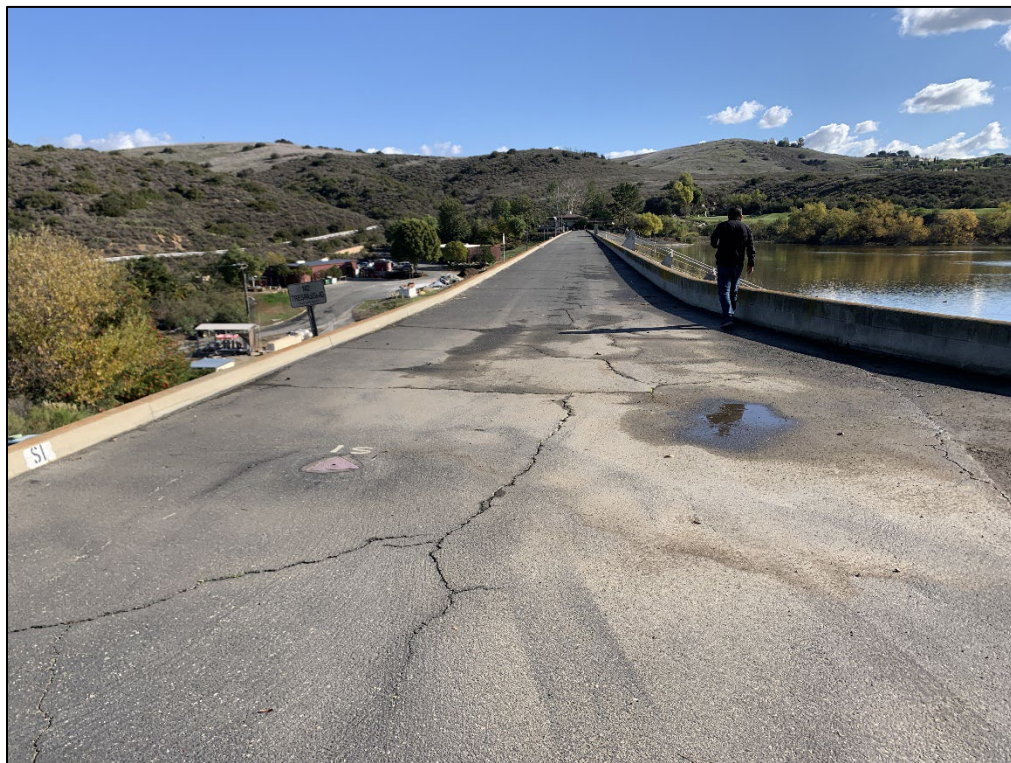
Photo 2) Minor AC paving cracking near left abutment looking towards the right abutment.
