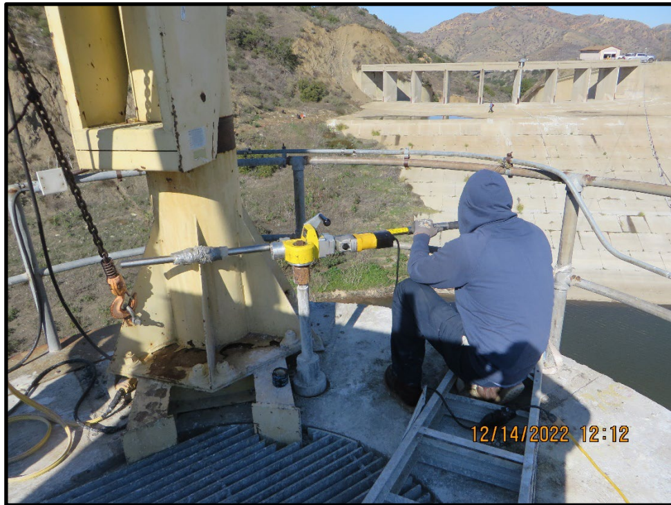
Photo 17) District exercising outlet gate valves at control tower.
