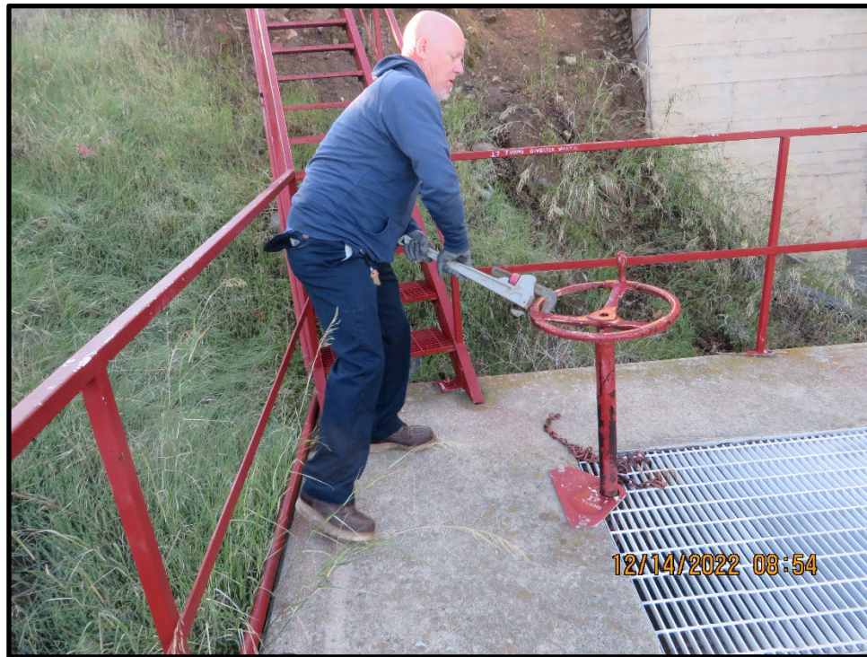
Photo 12) District exercising the emergency blowoff valve.
