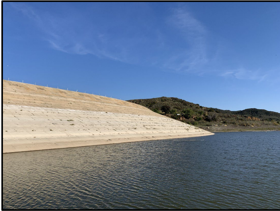
Photo 3) Upstream face looking towards right abutment. Note minor vegetation growing in cracks.
