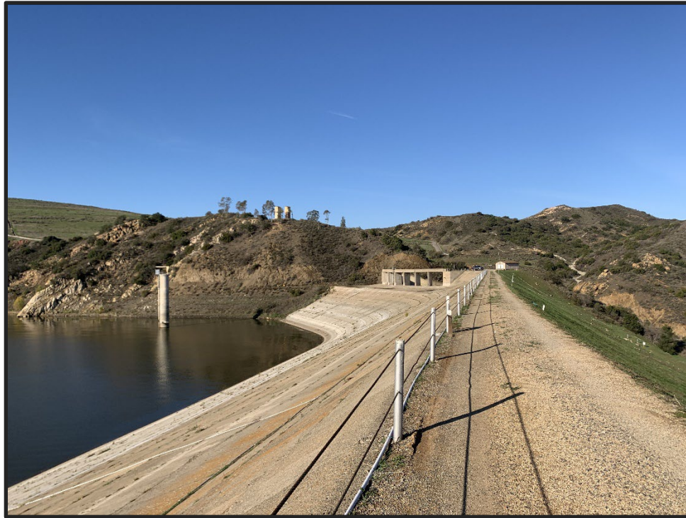
Photo 1) Dam crest, upstream, and downstream slopes. Note outlet tower and spillway approach.
