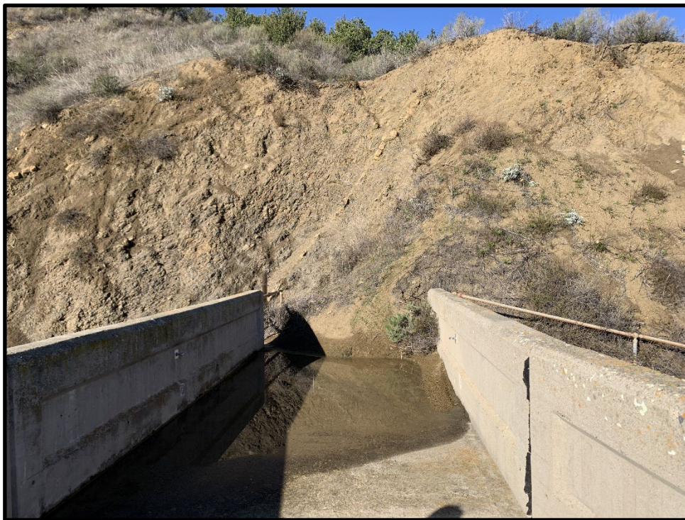
Photo 6) Close up sloughing from left abutment slope onto pedestrian bridge. Sloughing sediment has been cleared.
