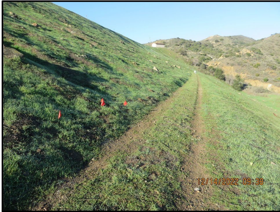
Photo 5) Downstream face bench looking towards left abutment. Note rodent control flag markings.
