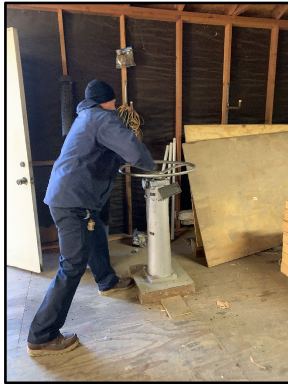
Photo 11) District exercising the downstream valve in control house.
