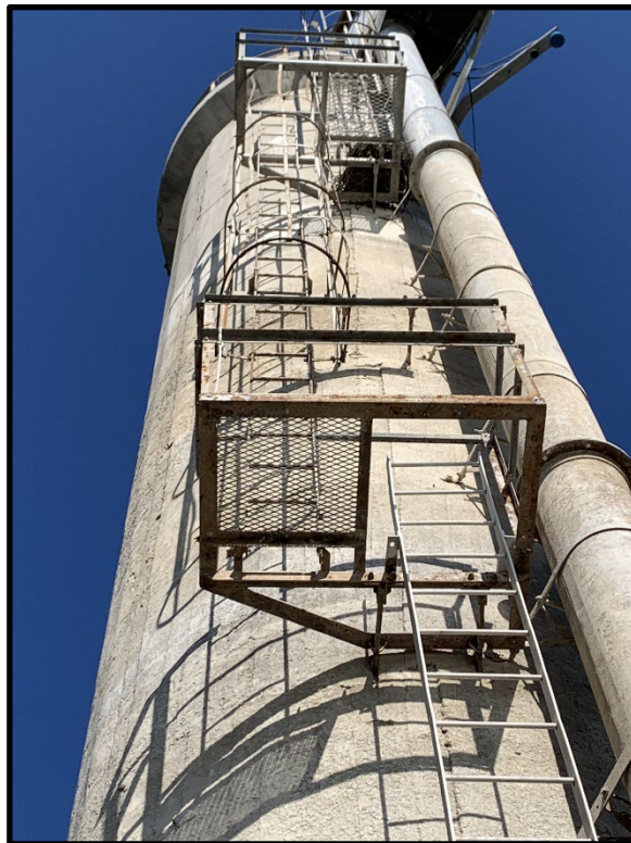
Photo 16) Access ladder for outlet tower. Note corrosion along ladder.
