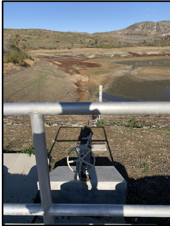
Photo 9) Outlet valve wheel and stem and reservoir staff gauge.
