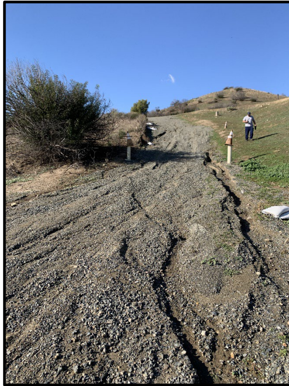
Photo 7) Minor rill erosion at right abutment access road
