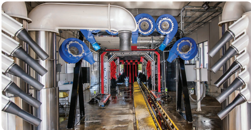
Inside the WaterStar-winning car wash.
