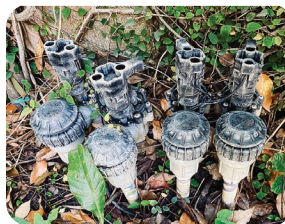
Old sprinkler valves
