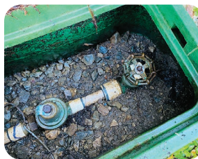
Irrigation shutoff valve
