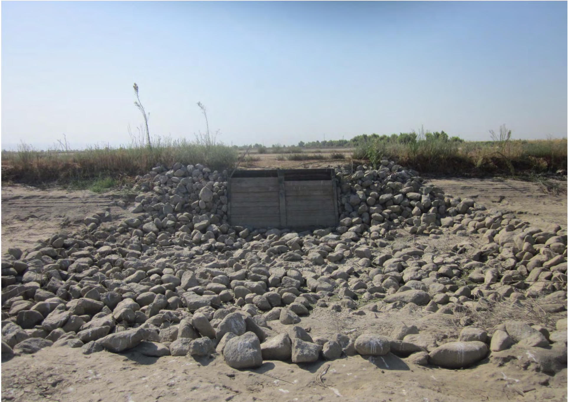
Photo 61 (22C): 2-Bay transfer structure between Basin No. 6 and No. 18
