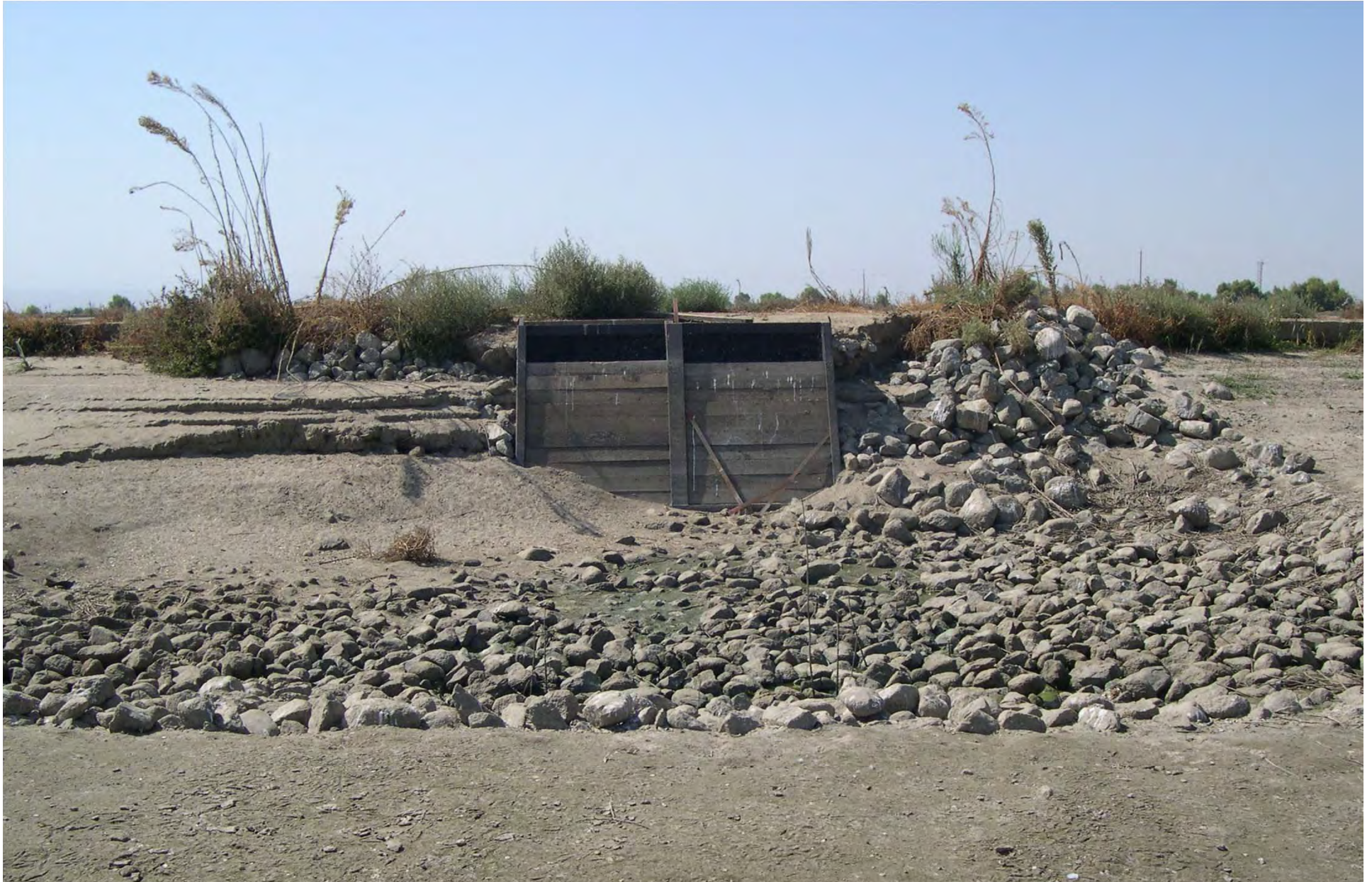
Photo 50b (15F): 2-Bay transfer structure between Basin No. 18 and No. 19; sediment covers part of rip-rap and outlet structure; green algae mat covers sediment adjacent to rip-rap; west berm erosion
