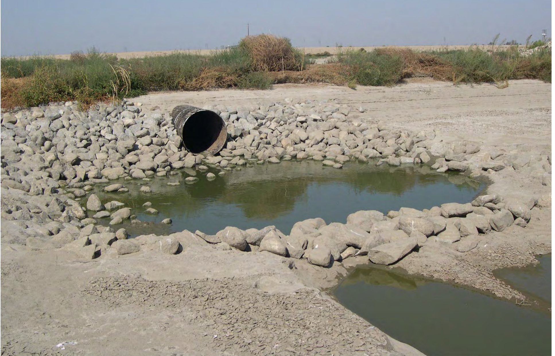
Photo 57b (23E): 1-Bay transfer structure between Basin No. 6 and No. 3; stagnant water with algae in rip-rap; small wash-out adjacent to rip-rap
