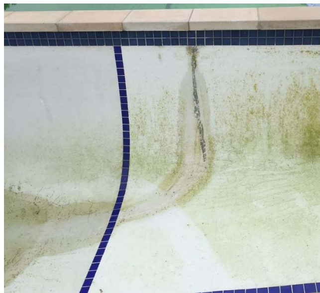
FIGURE 10: LEAKAGE FROM POOL 3 TO POOL 4
