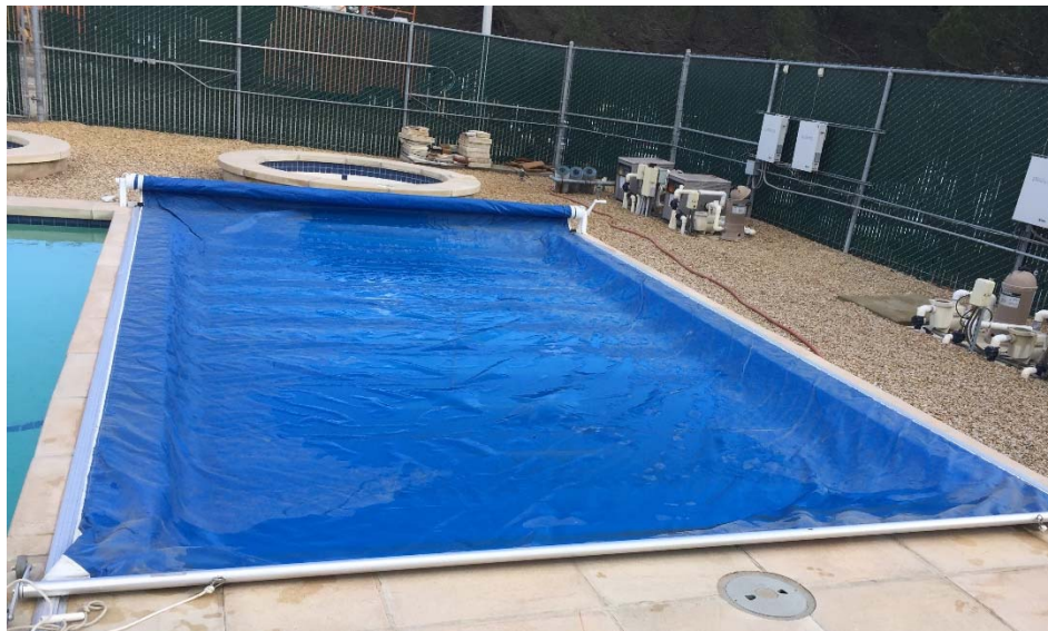
FIGURE 1. SOLID TRACK COVER MOUNTED TO A POOL AT THE NPIRC
