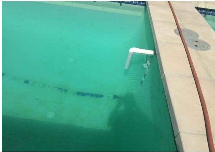
FIGURE 9. A SYPHON INSTALLED IN POOL 1
