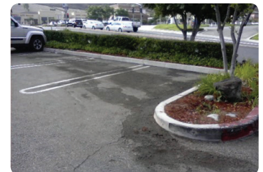
Asphalt erosion caused by runoff.
