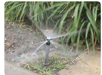
Broken spray head.
