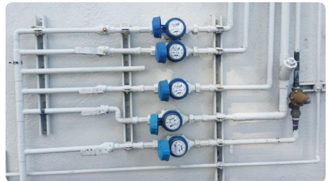
The use of submeters improves water efficiency and the ability to locate leaks.
