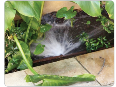
Broken drip line.
